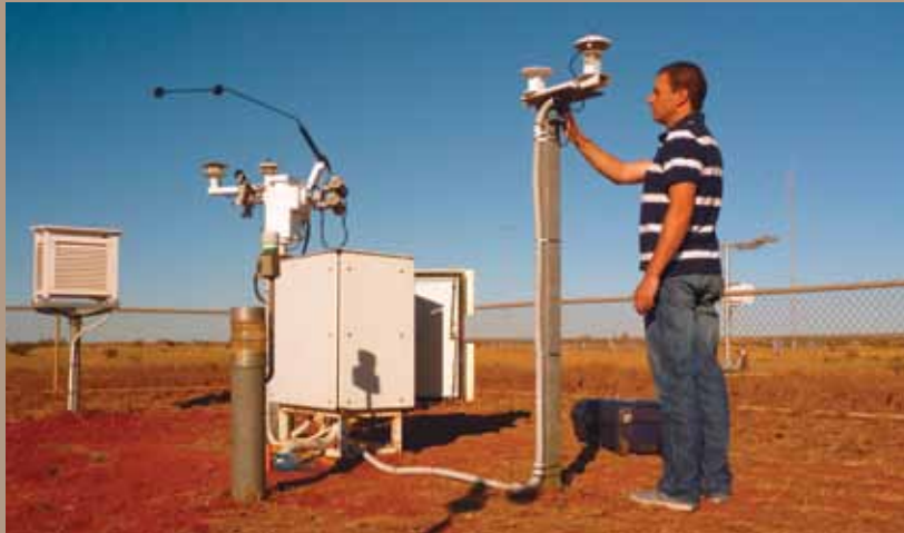
Bureau of Meteorology technician Paul Freeman inspecting solar radiation monitoring equipment after its recent installation in Learmonth, Western Australia
